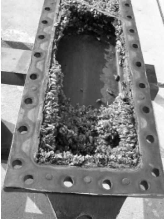
Fig. 2. Macrofouling of Limnoperna fortunei into the water distribution systems of Palmar hydroelectric power plant.
